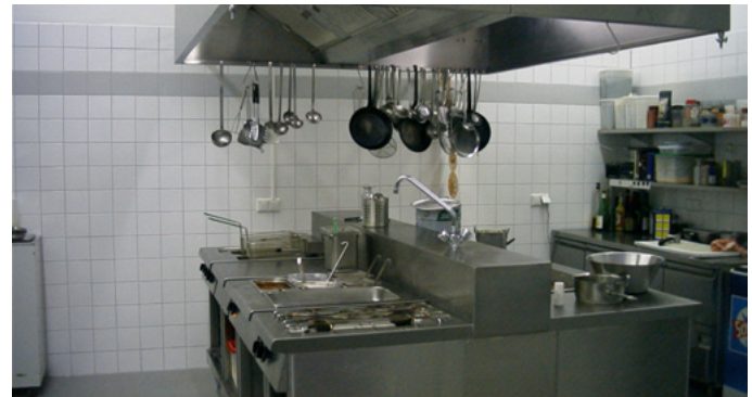
Filter monitoring in kitchens
